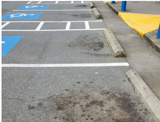
Photo 2: Stained parking spaces
